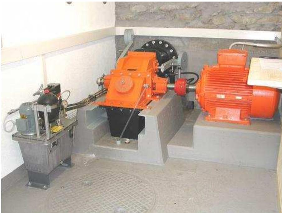
Figure 3: Crossflow turbine with generator and hydraulic pump for valve actuators
